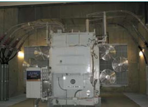
A 69kV/12kV transformer is labeled for visitors to the showcase Park Substation in Anaheim, California.
