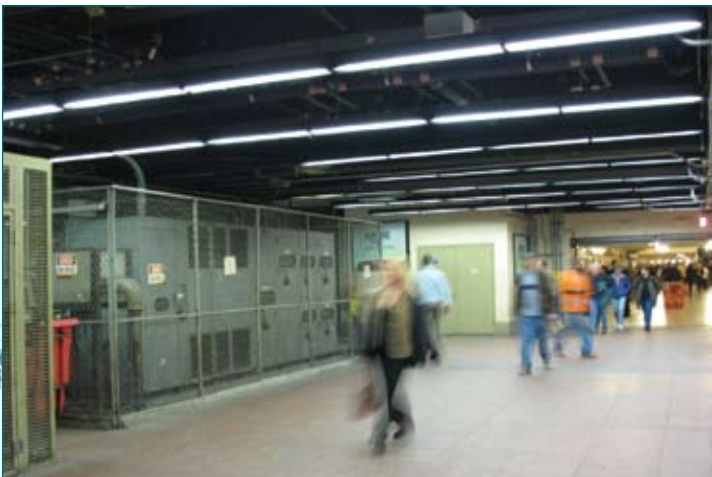
Each day, thousands of New York commuters stream past exposed 13.2kV transformers without a second glance.
