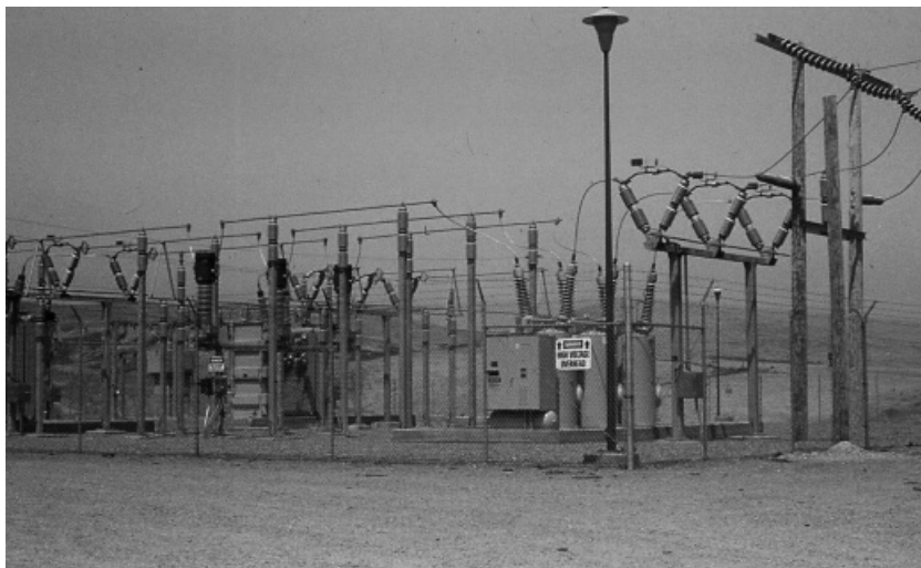
Figure 6.10 Distribution substation. (Courtesy of Marshal F. Merriam.)
