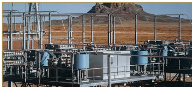
figure 1. Western Area Power Authority Kayenta Substation (165 MVAR TCSC/230 kV).
