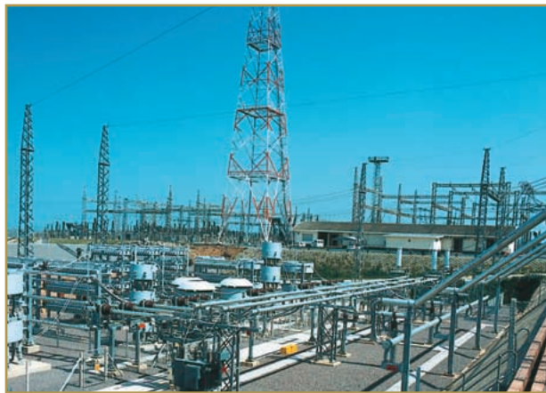
figure 2. A typical example of a static VAR compensation installation.
