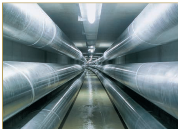
figure 4. A gas insulated transmission line tunnel in Switzerland.
