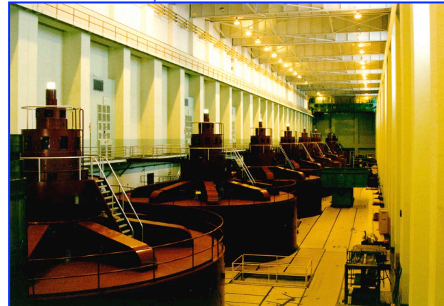
Hydroturbine-generator units at Grand Coulee Dam, each unit \approx 50MW
