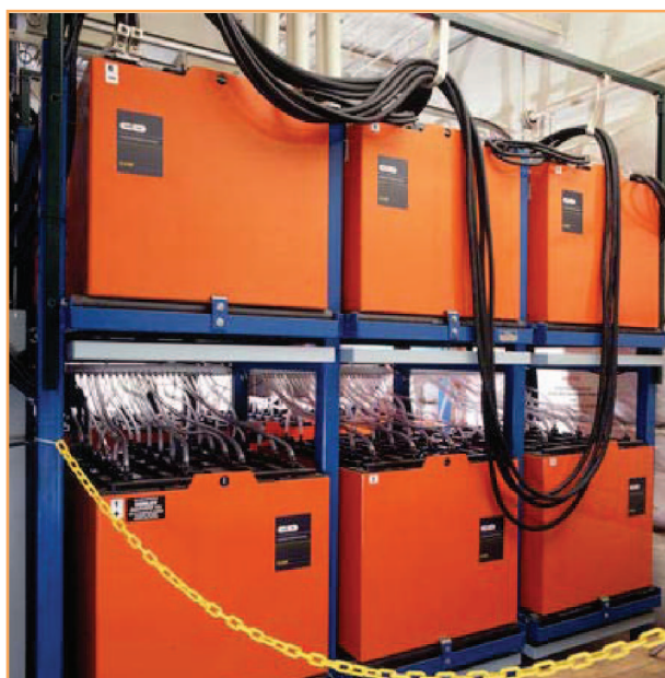
figure 6. Large lead-acid battery bank.
