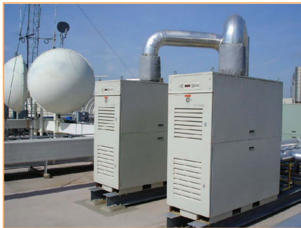
figure 2. Microturbines with heat recovery.
