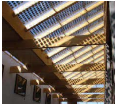
A photovoltaic array integrated onto the roof atrium of the student services building at Southampton University © University of Southampton
